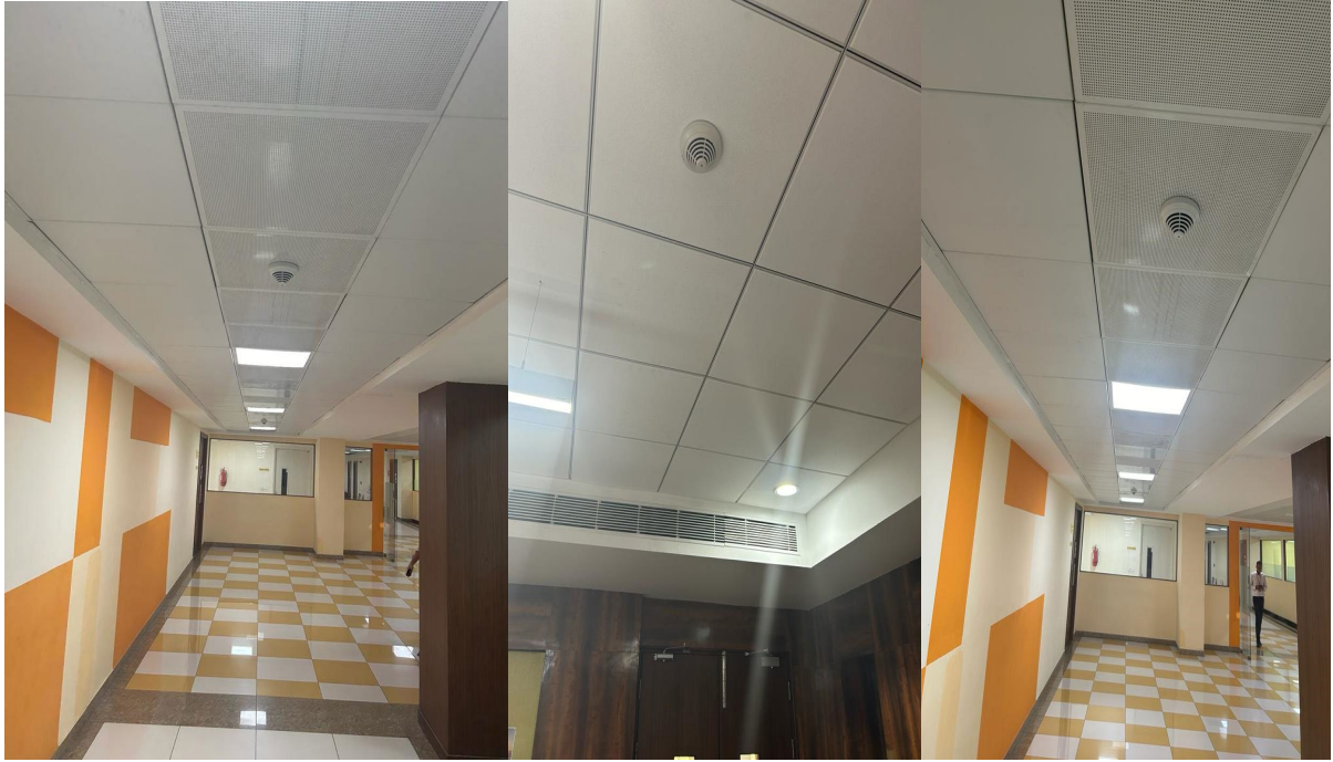
Picture 3: Smoking alarms and detectors installed in MUJ to ensure No Smoking in the campus
